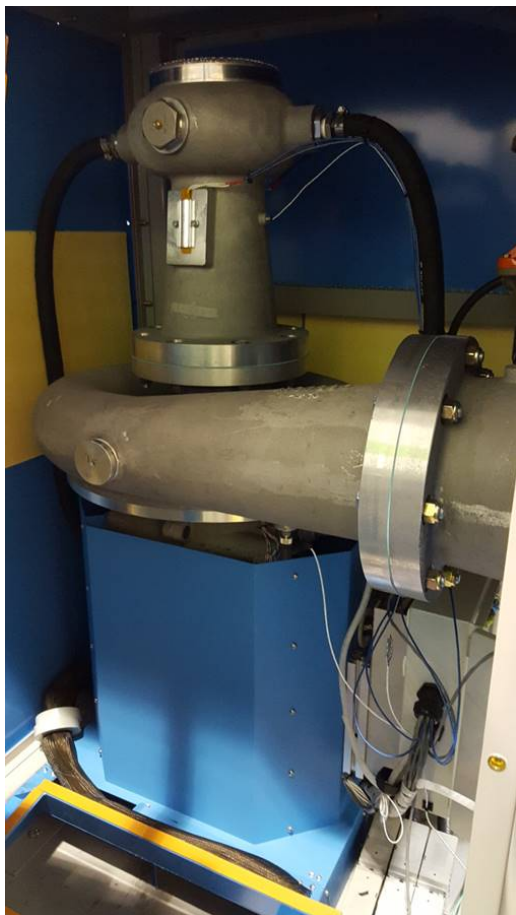
Fig. 17: Core machine installed in cabinet with inlet venturi and cooling shroud.
